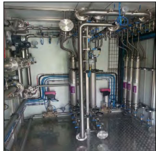
Local membranes (Source : Clarke Energy)
